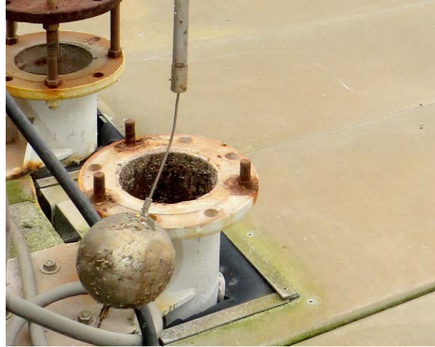
Figure 08. Float Switch Damage Bent float support rod.
