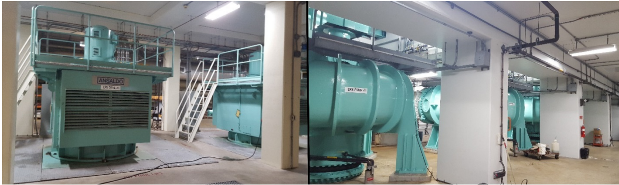
Figure 05. Effluent Pump Station
