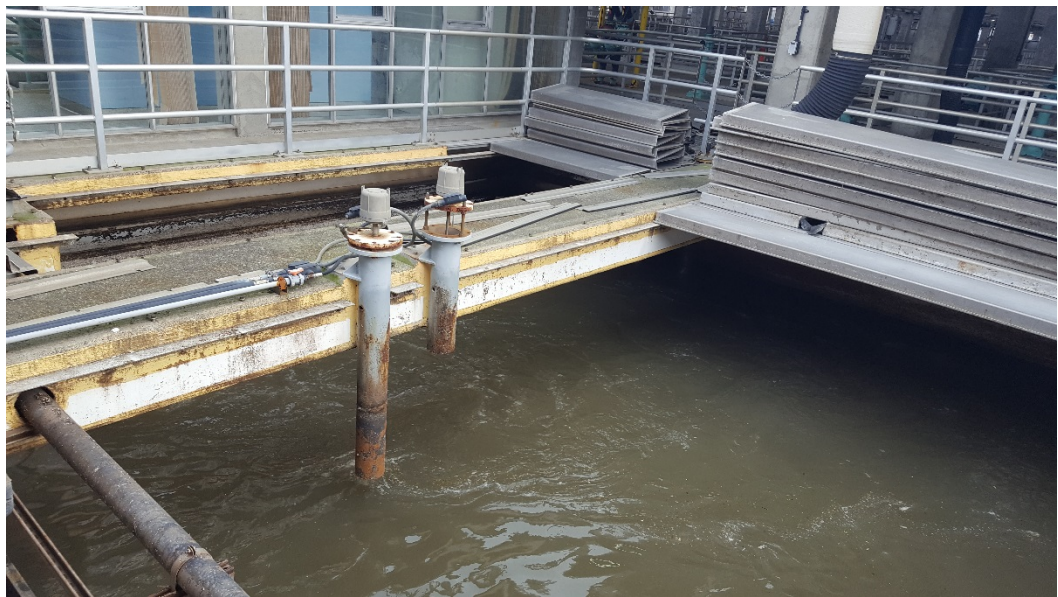
Figure 10. Float Switch Location
