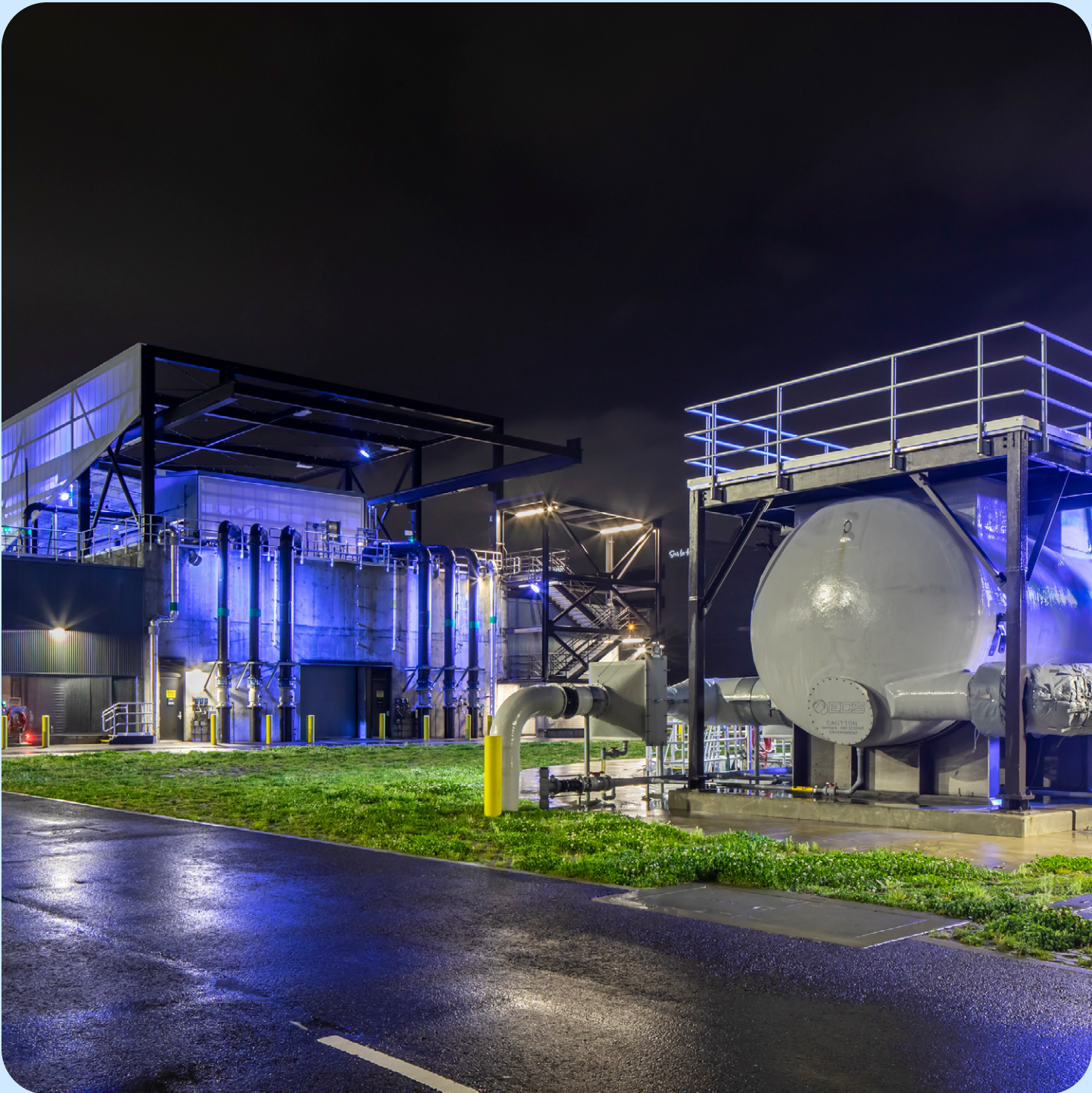
King County's Georgetown Wet Weather Treatment Station, located in Seattle's Georgetown neighborhood. The station was designed to account for two feet of sea level rise.
