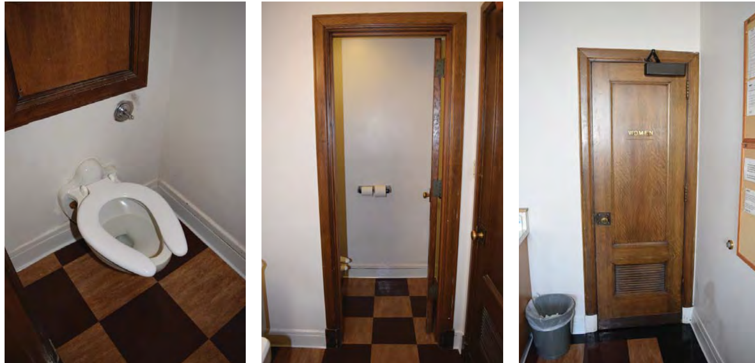
King County Courthouse typical non-ADA compliant jury deliberation room restroom and door. CDG photos, May 20, 2016.
