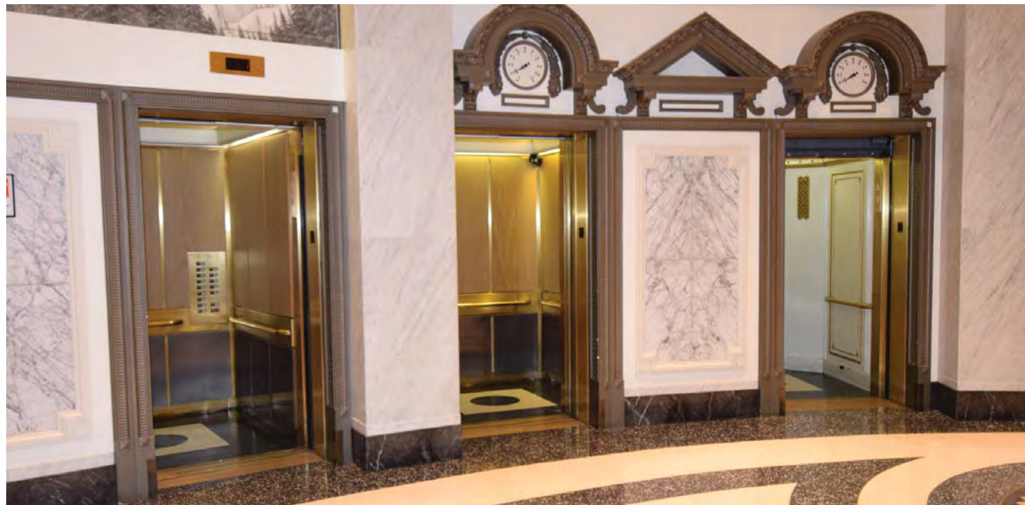
View of elevators on fire service recalled to level 1 during inspection. CDG photo, April 16, 2016.
