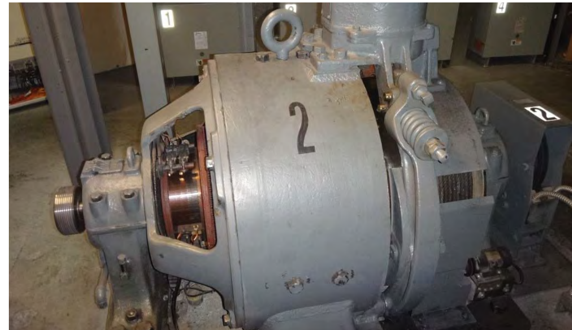
Figure 2 – Original Westinghouse Gearless machines for Cars 1-10 appear to have been installed during the 1960 modernization of the Court.
