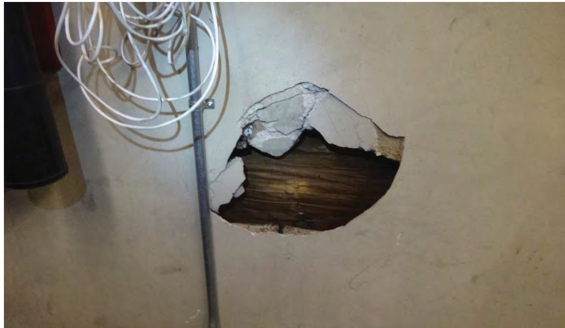
Figure 4 – Hole in the wall of the elevator machine room.
