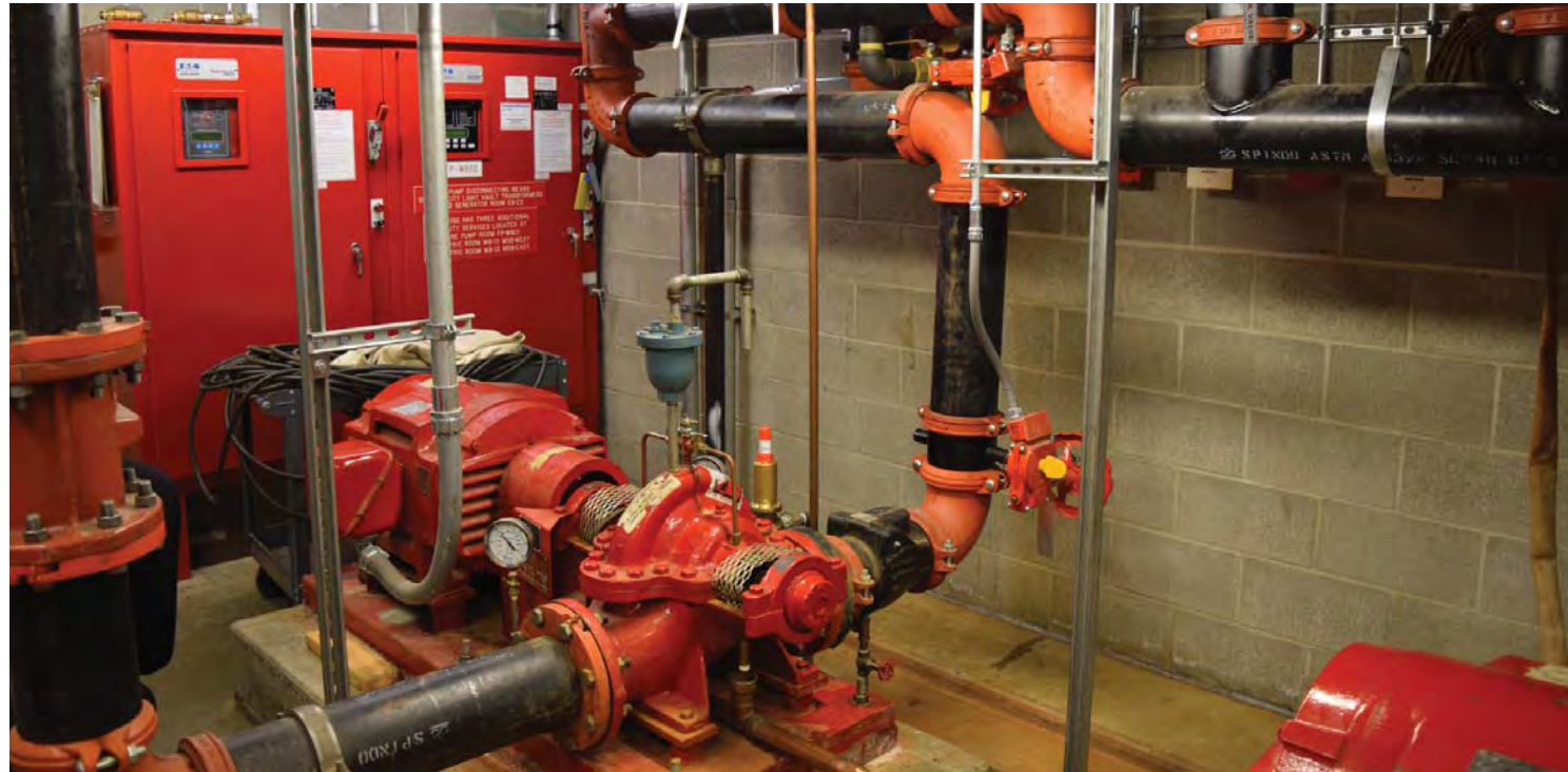
Photo of fire sprinkler pumps, fire sprinkler control panel, and fire protection water piping at basement Room WB9B. CDG photo, May 24, 2016.
