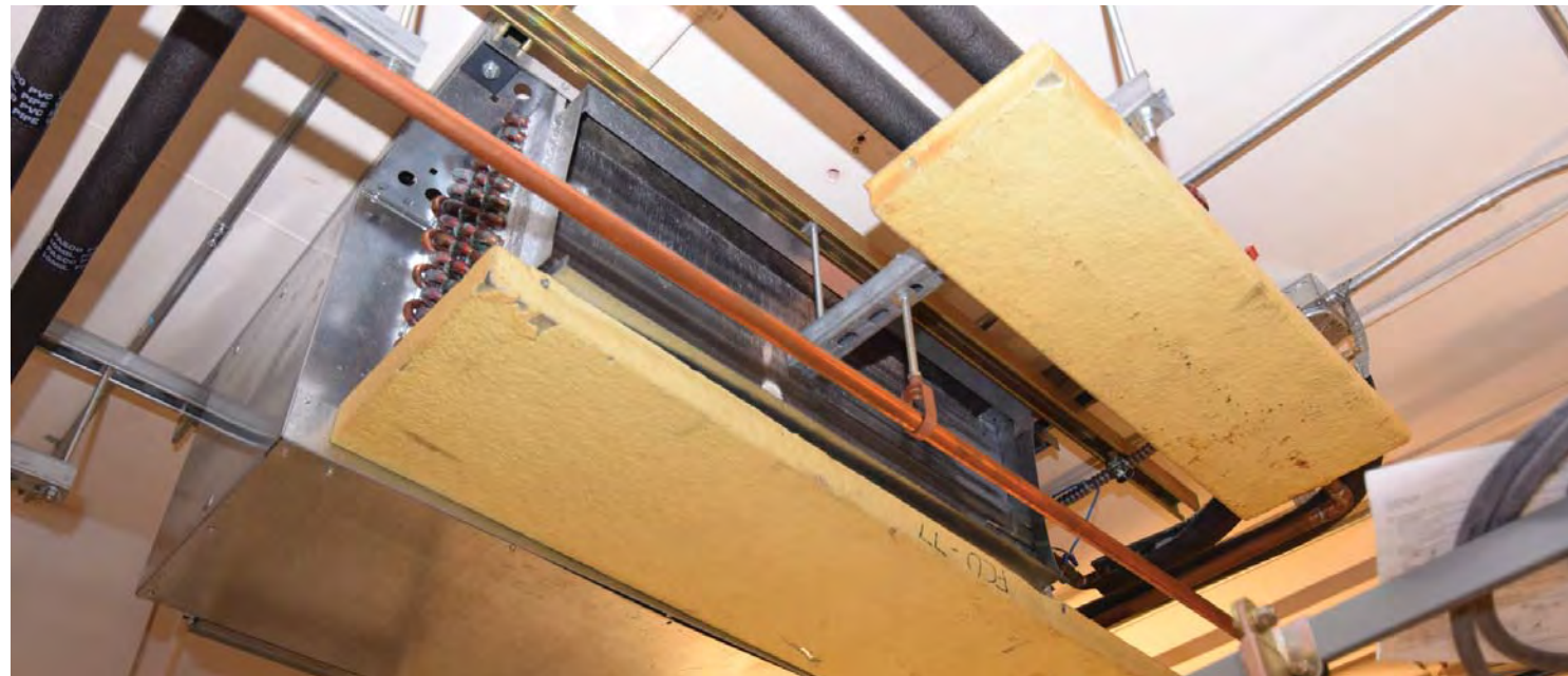
Fan Coil Terminal Units
