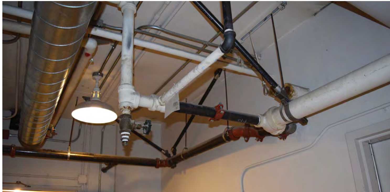
View of seismic bracing for fire protection water piping at ceiling of basement Room EB9. CDG photo, May 24, 2016.
