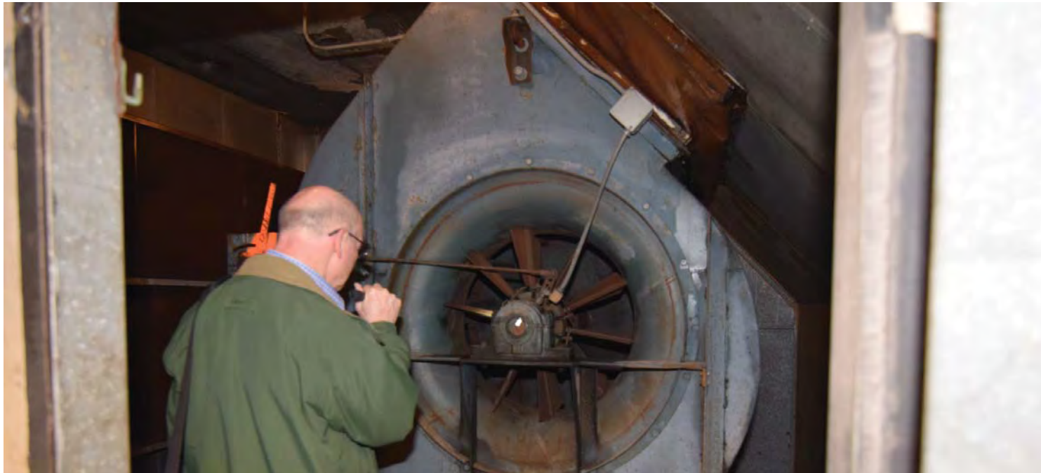
Air Handling Unit
