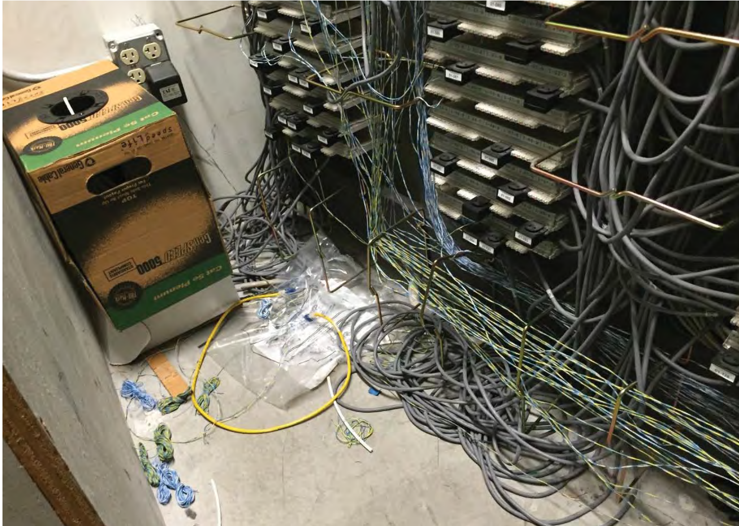
FIGURE 12 Proprietary low-density cable patching system. Debris from construction and maintenance has been allowed to accumulate in communication spaces
