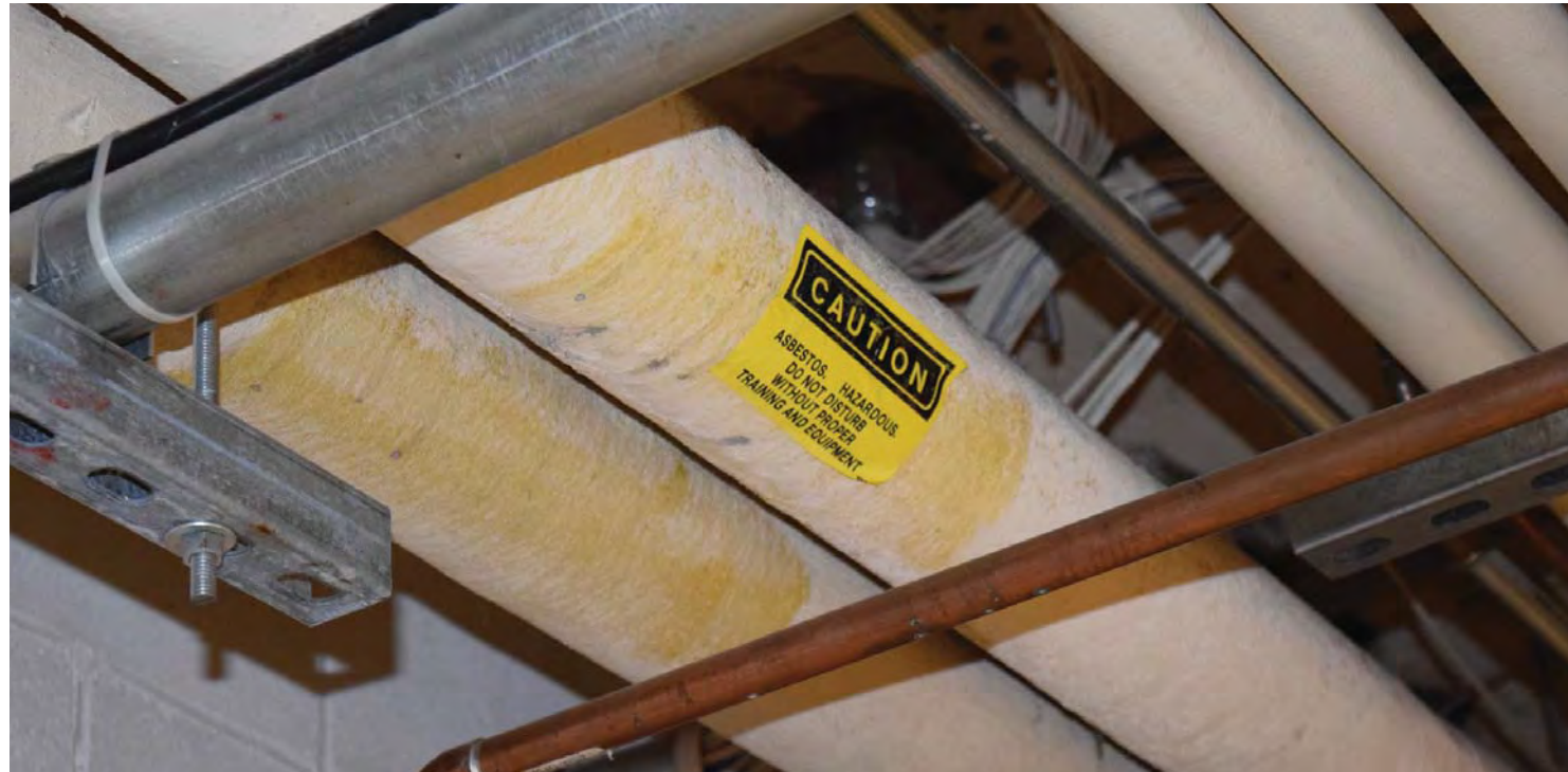
View of label identifying asbestos pipe insulation. CDG photo, May 24, 2016.
