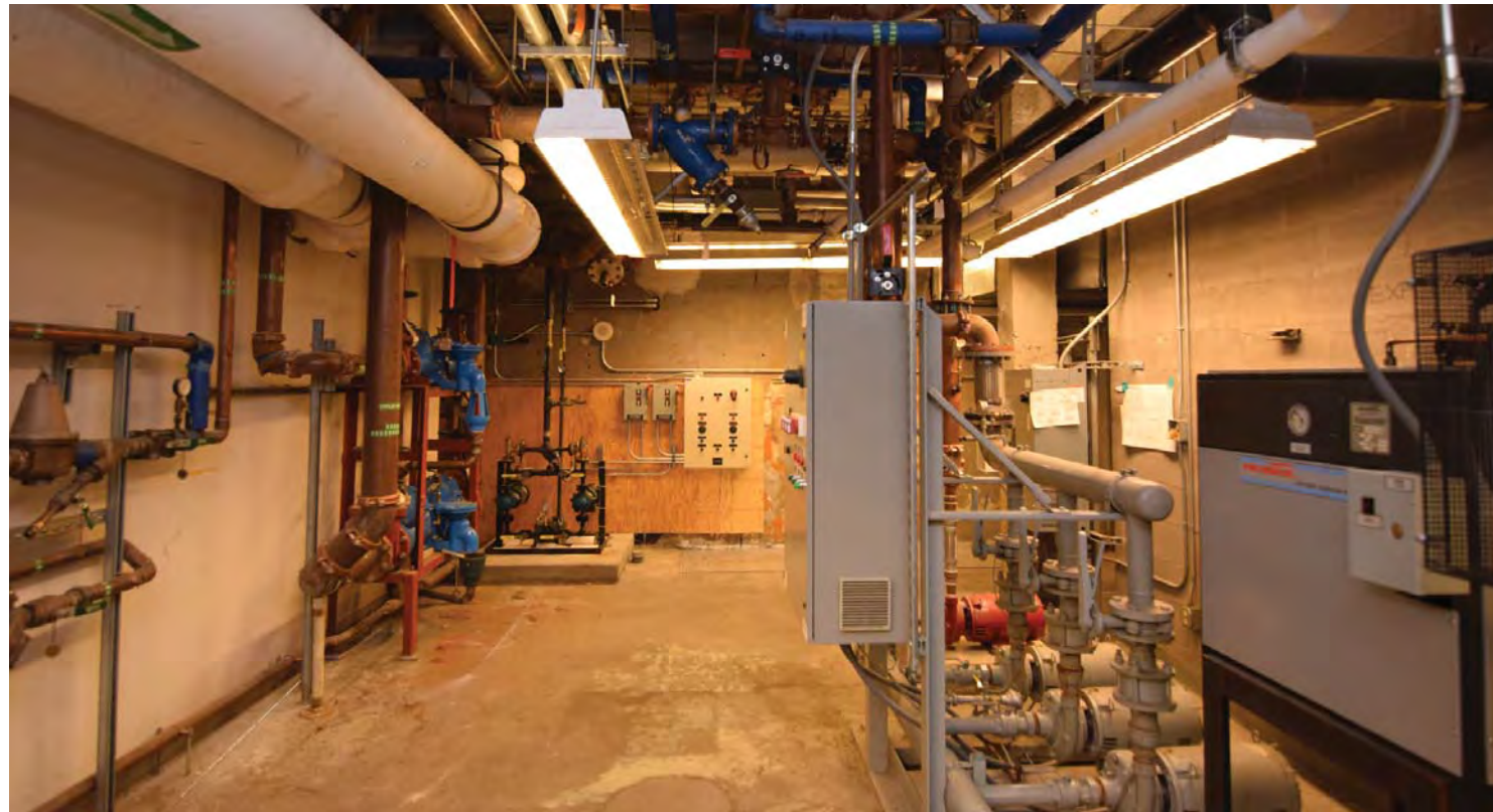
Domestic Cold Water Booster Pumps
