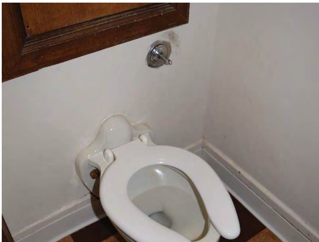
King County Courthouse interior view of plaster wall finish at jury deliberation room restroom W727B. CDG photo, May 20, 2016.
