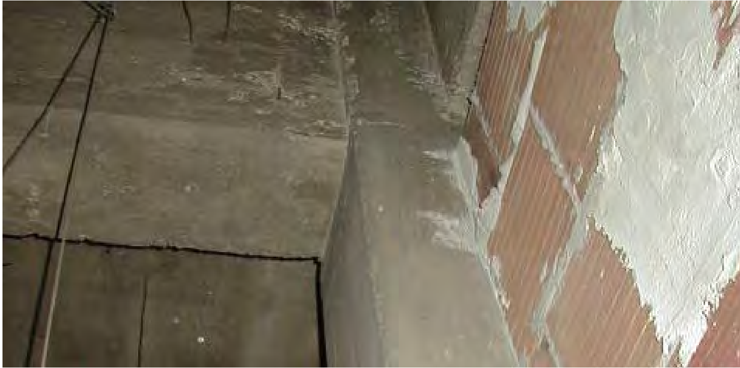
King County Courthouse, view of hollow clay tile infill between reinforced concrete columns at exterior walls. CPL photo, February, 1, 2001.
