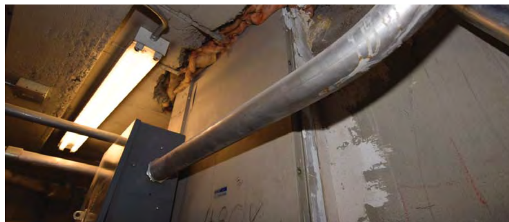
Bus duct photo
