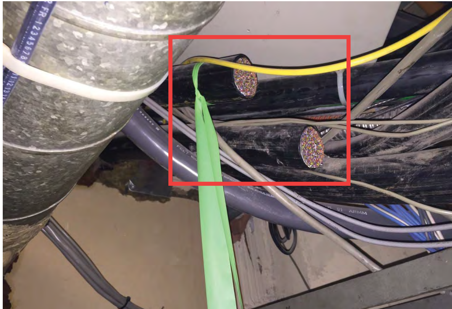
FIGURE 8 Communication cables have been severed and abandoned in place
