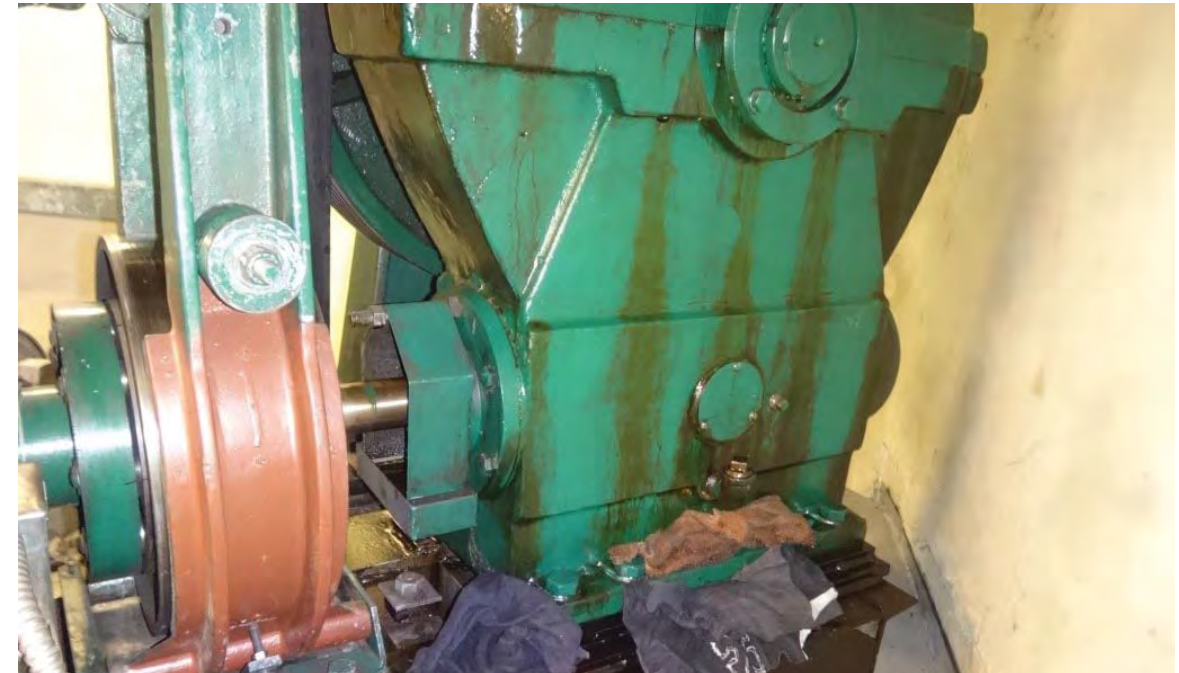
Figure 5 – Geared elevator machine for Cars 11 and 14 is leaking oil.
