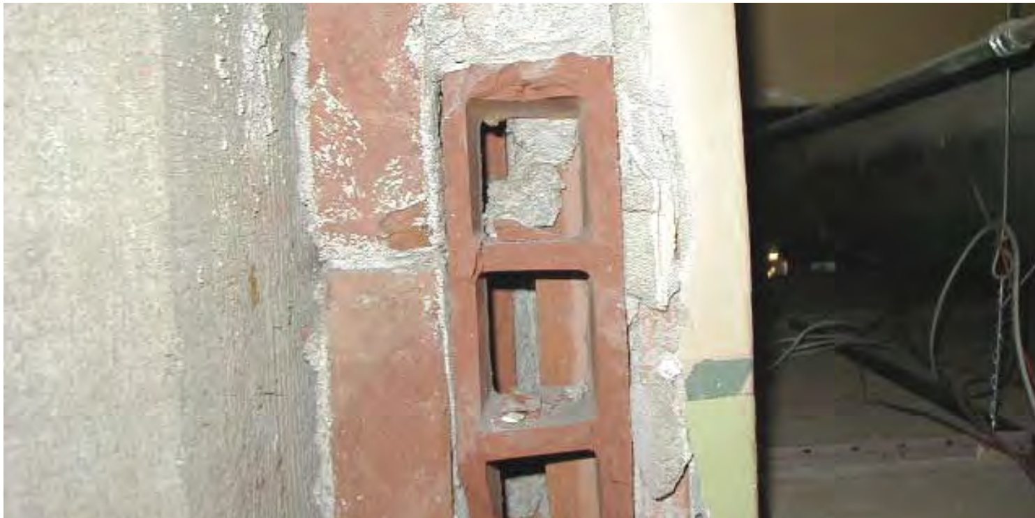
King County Courthouse, detail view of voids inside hollow clay tile infill at exterior walls. CPL photo, February 1, 2001.
