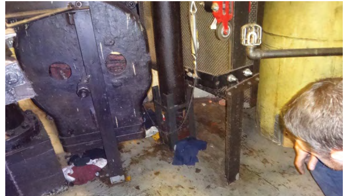
Figure 14 – Typical pit with rags and dirty floor.
