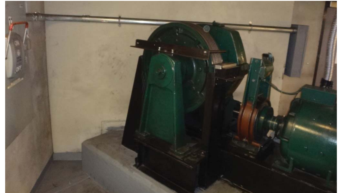
Figure 13 – Geared hoist machine for Car 11. Manufactured by Dover.
