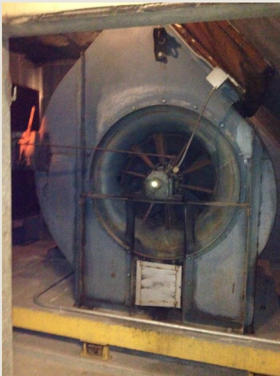
Figure 6 1965 era Dual Duct Single Fans
