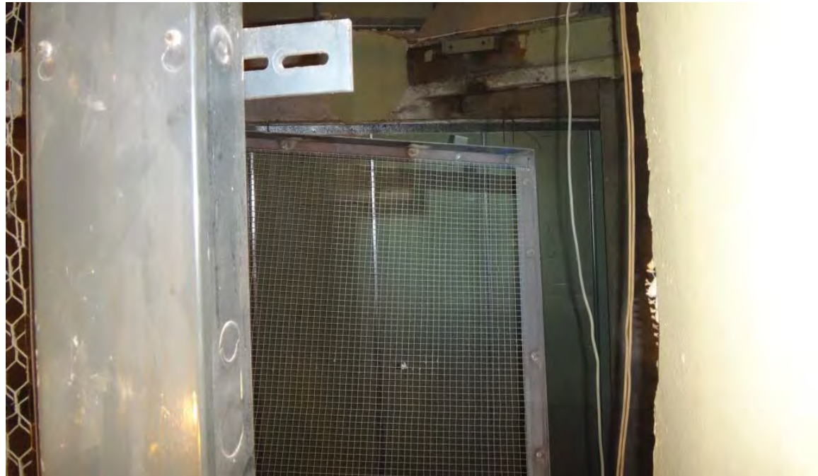
Figure 11 – Part of hoistway screening between Cars 9 and 10 is coming down and should be re-anchored.
