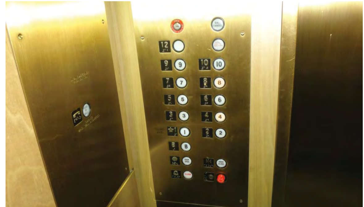
Figure 6 – Bronze fixtures installed in 2004/5 during modernization Meet code except for push/pull stop switch.
