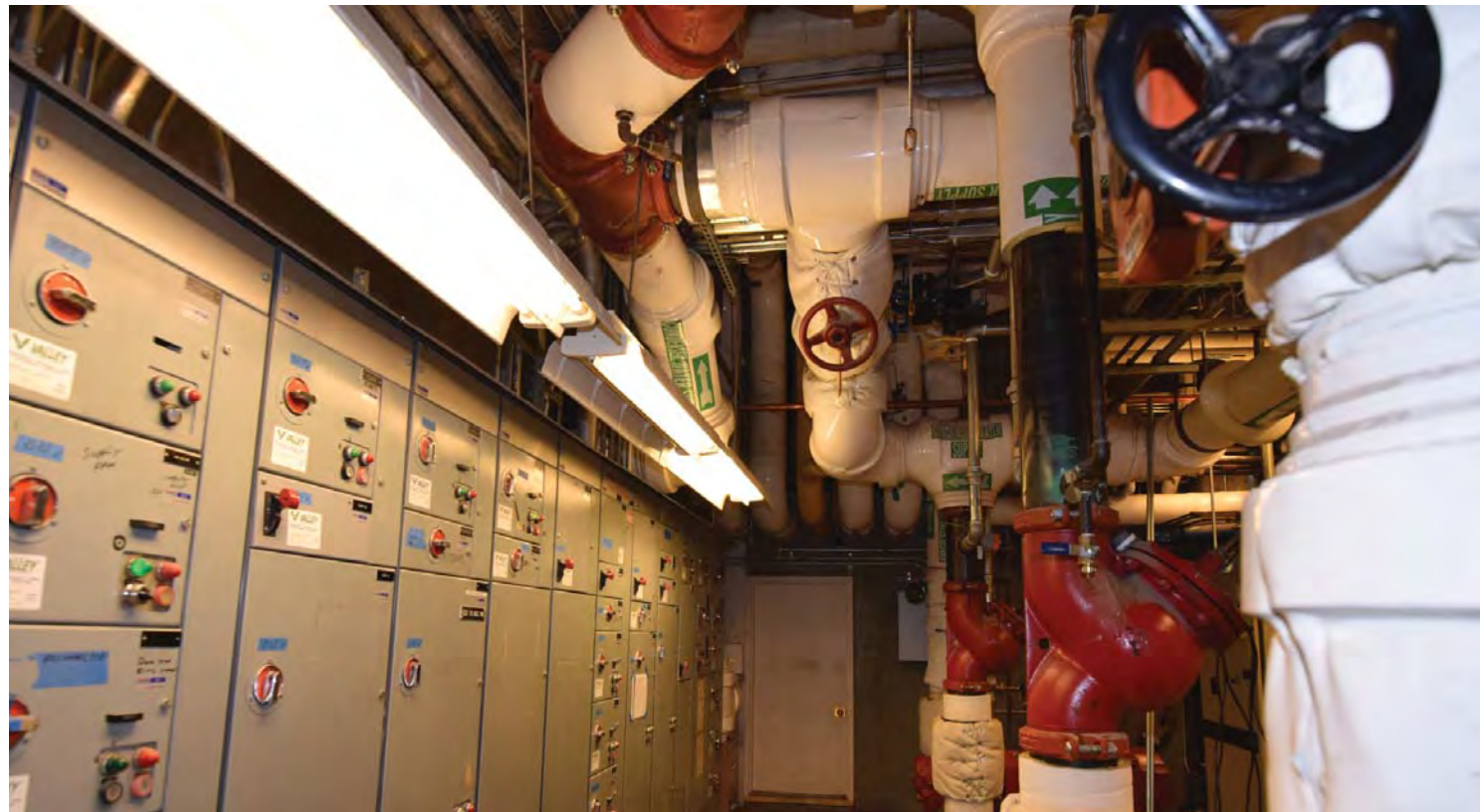
One of the existing motor control centers
