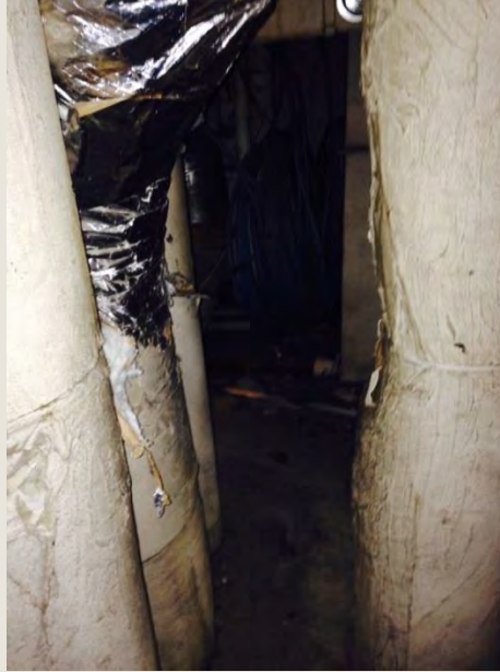
Figure 3 Access to floor 1A east electrical room (part two) by crawling through an 8” wide space between heating riser pipes. Extracting an injured worker from behind here would be next to impossible.
