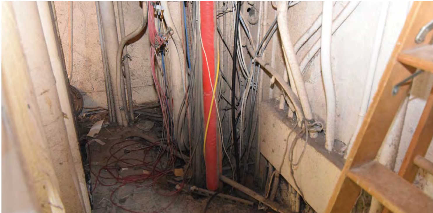
View of space inside vertical mechanical, electrical, and plumbing shaft. CDG photo, May 31, 2016.
