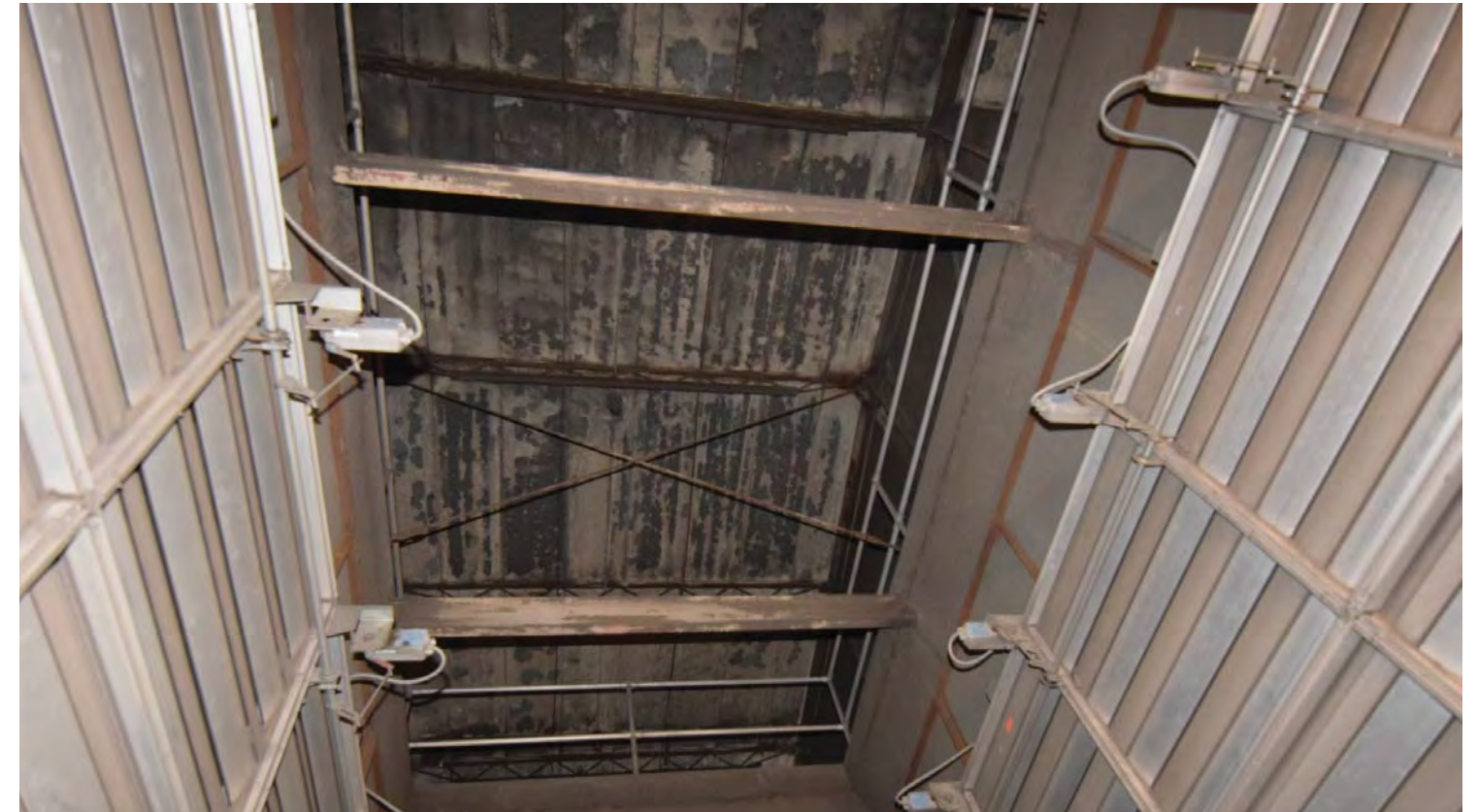
Outside Air Intakes
