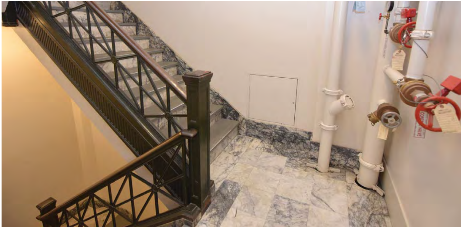
Photo of Stair 4 at level 5. The existing handrail is non-code compliant and may need to be upgraded if the building is substantially altered. CDG photo, May 7, 2016.
