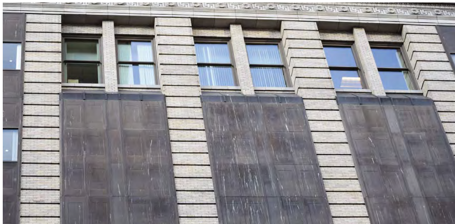
King County Courthouse exterior, detail view of the aluminum window wall systems at the Fourth Avenue facade. CDG photo, March 18, 2016.
