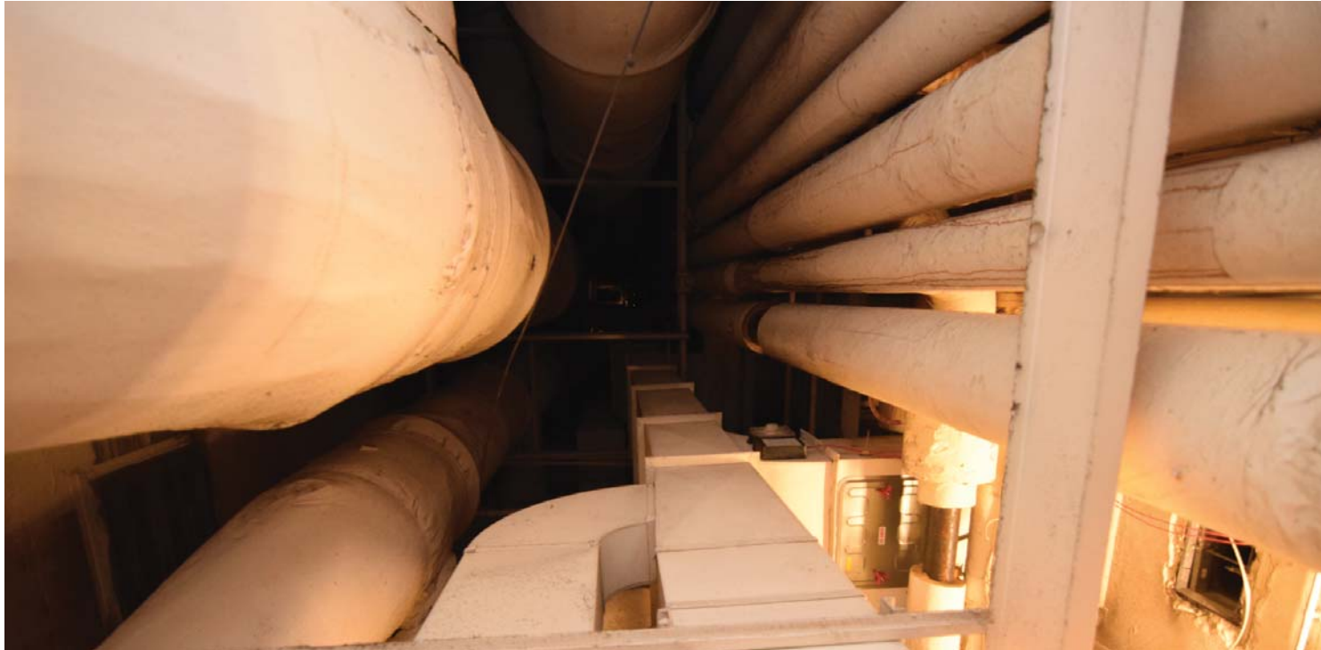
View of ducts and piping inside vertical mechanical, electrical, and plumbing shaft. CDG photo, March 31, 2016.
