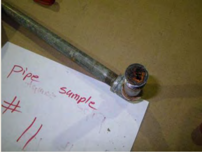
Figure 4 Pipe Sample from Courthouse domestic water system
