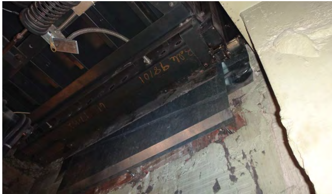
Figure 12 – Car aprons are missing from most of Cars 1 to 10.
