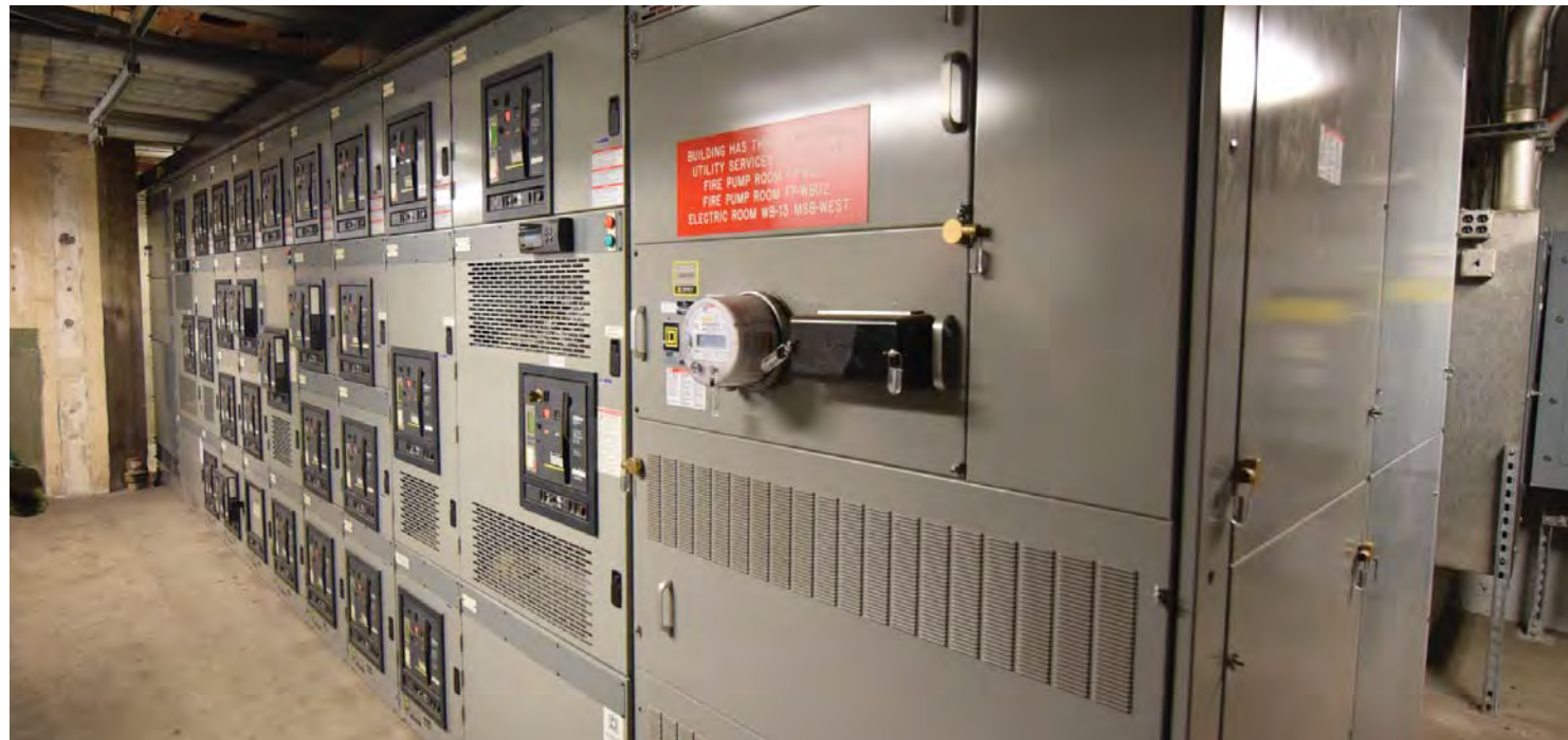
Main switchboard photo
