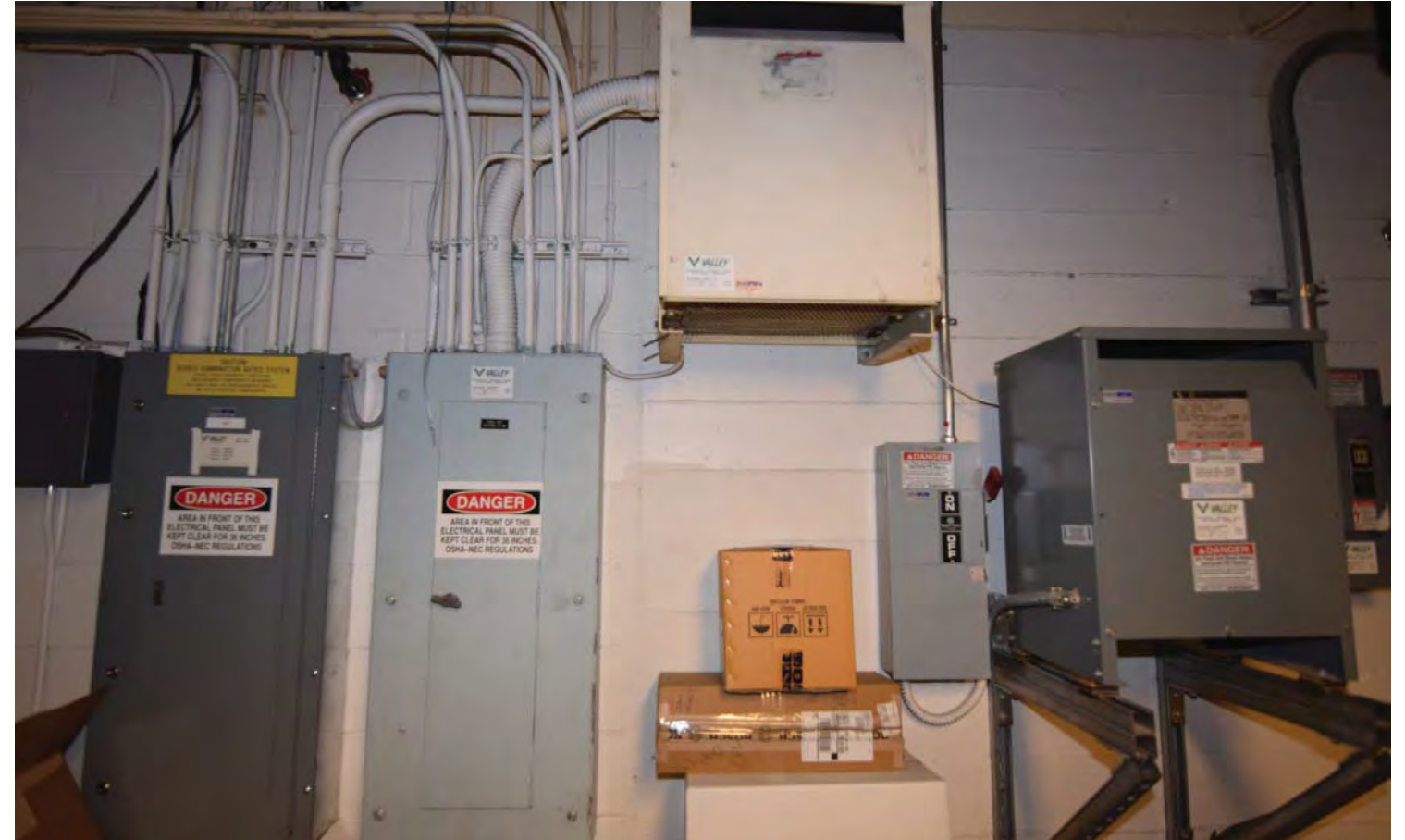
208V circuit breakers
