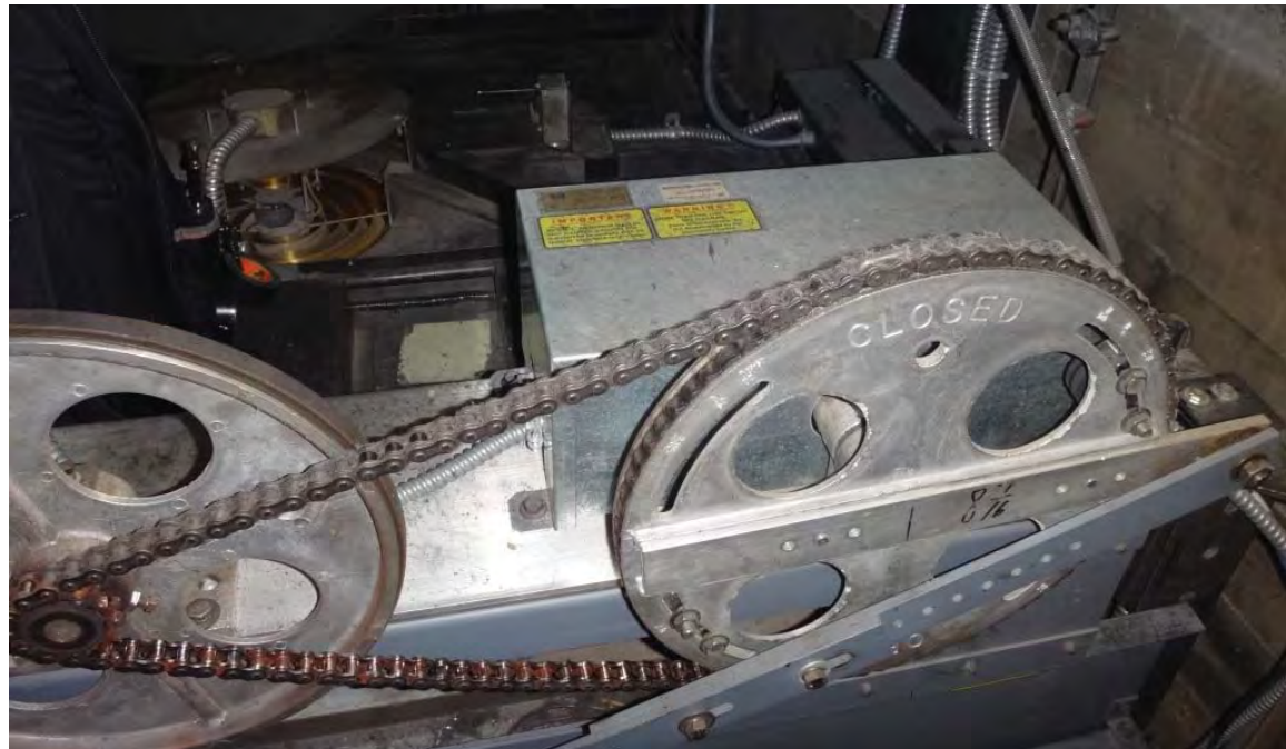
Figure 8 – GAL MOVFR closed loop door operators installed during modernization in 2004/5.
