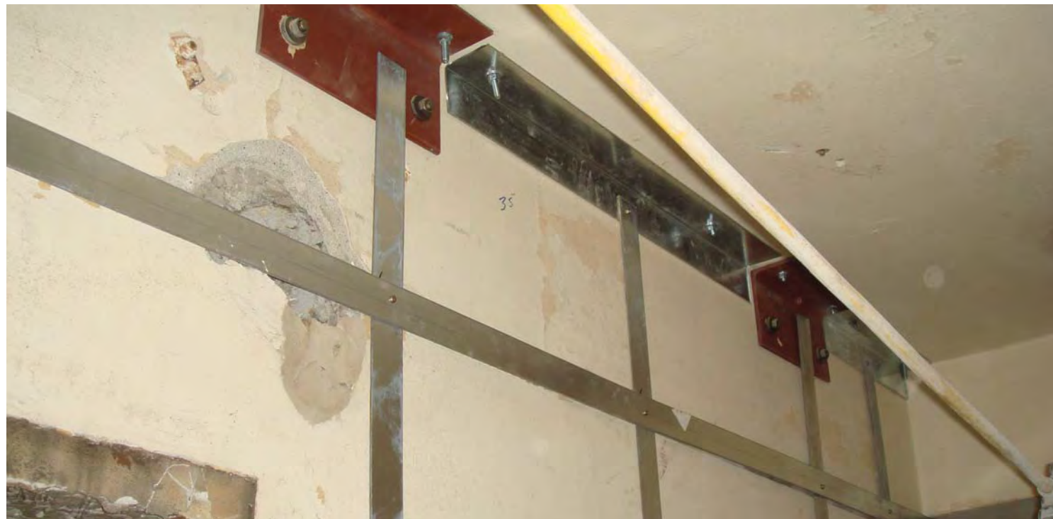
Example of steel strap strongbacking for hollow-clay tile masonry interior wall. CDG photo, April 22, 2015.
