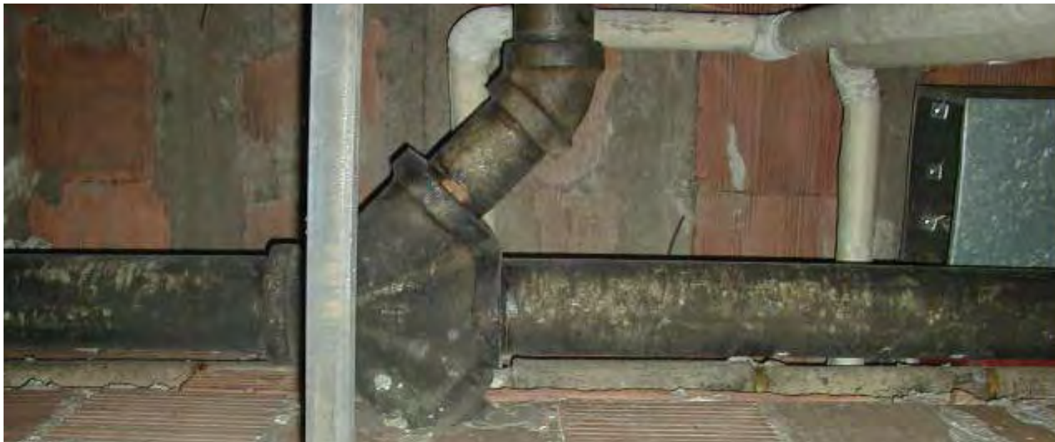
Cast-iron sanitary waste piping. CPL photo, February 13, 2001.
