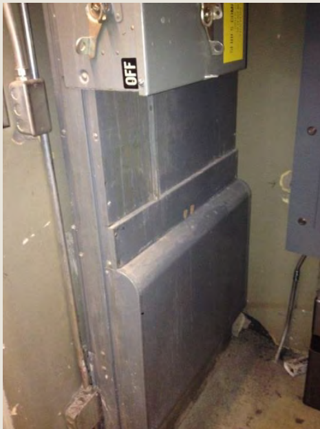
Figure 1 4000 amp buss electrical buss duct (East Riser)
