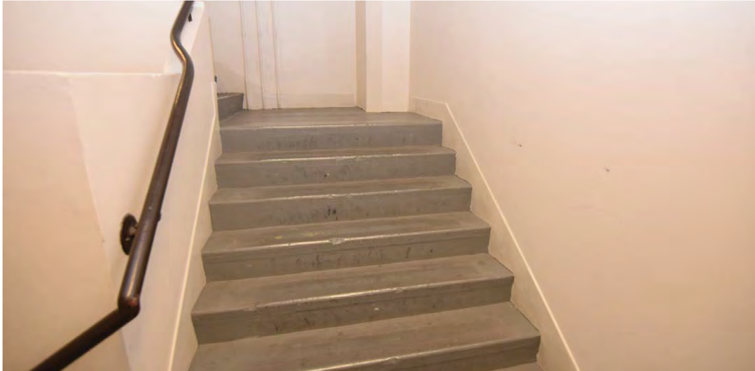
Photo of Stair 4 at level 10. A handrail would need to be added to the stair if the building is substantially altered. CDG photo, May 7, 2016.
