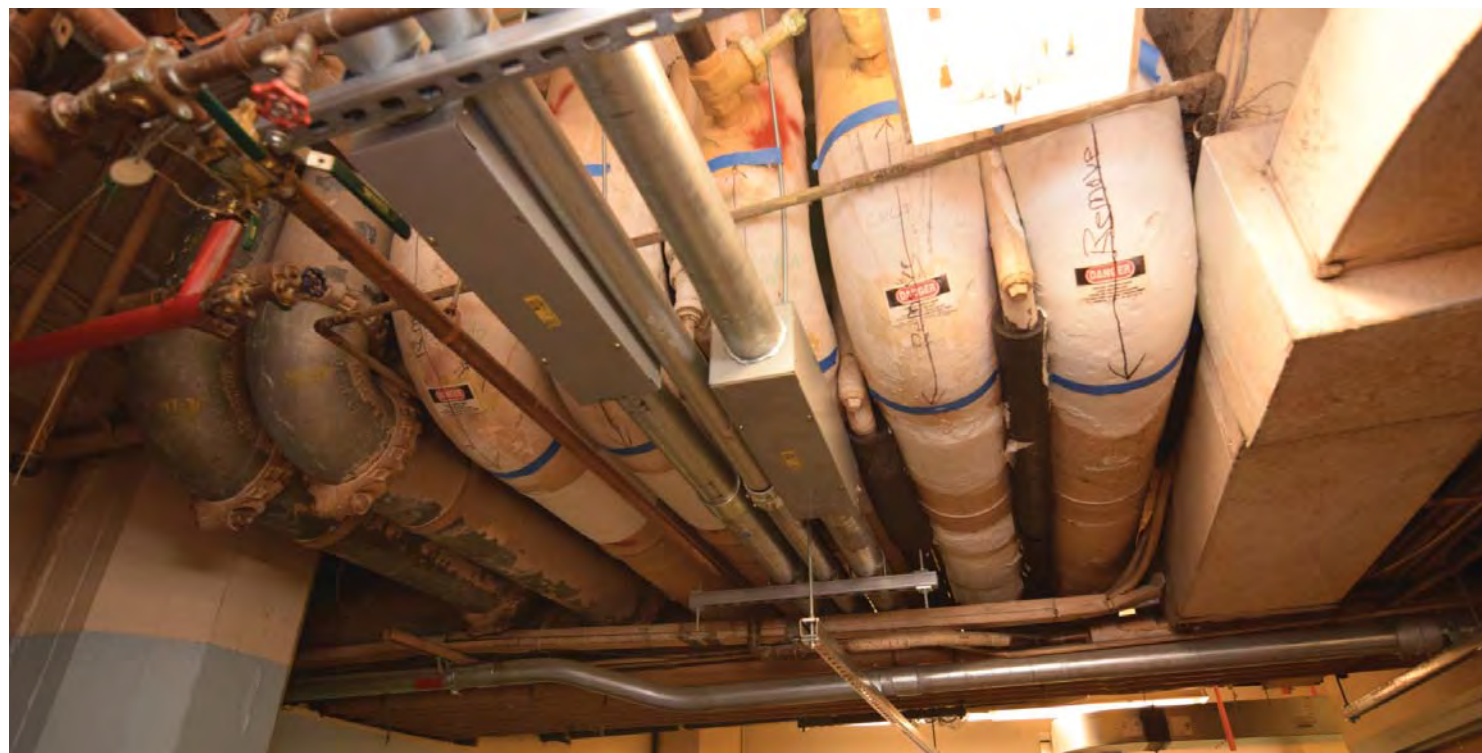
View of labels identifying asbestos pipe insulation. CDG photo, March 18, 2016.
