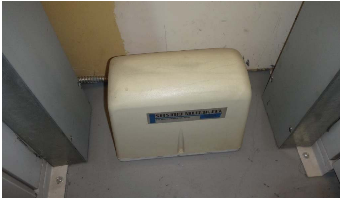
Figure 3 – Seismic switch installed during the modernization in 2004/05.
