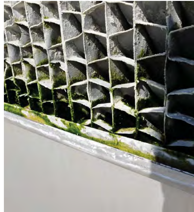
Cooling Tower close-up
