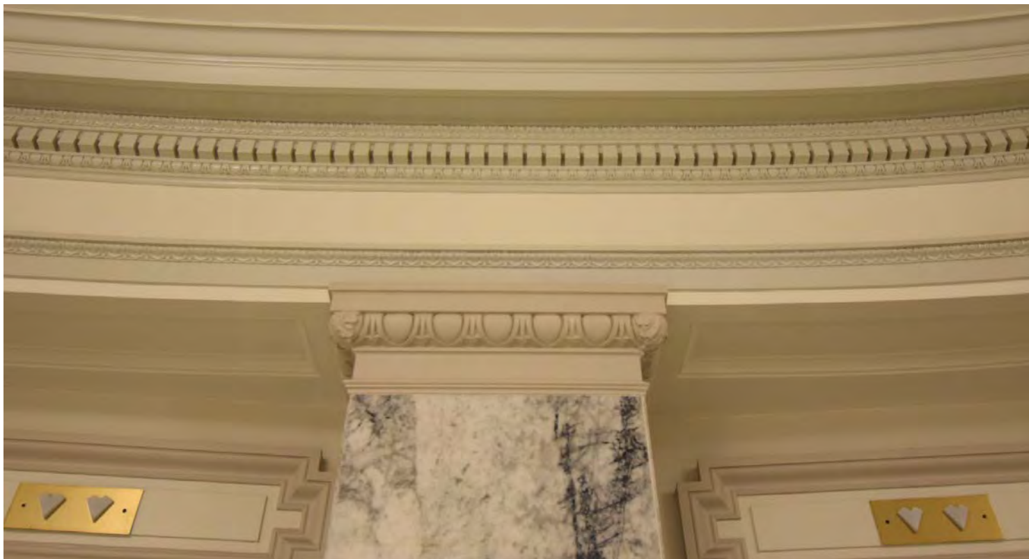
Detail of plaster molding at ninth floor elevator lobby. CDG photo, April 16, 2016.
