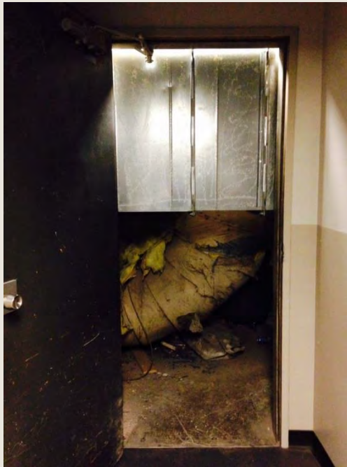
Figure 2 Access to floor 1A east electrical room by crawling under ductwork, a serious safety hazard and code violation
