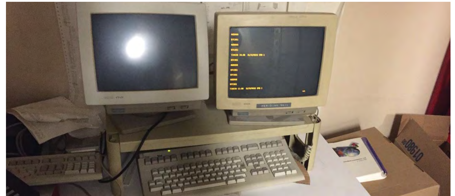
FIGURE 6 Obsolete voice-mail server terminal, consuming power and generating heat
