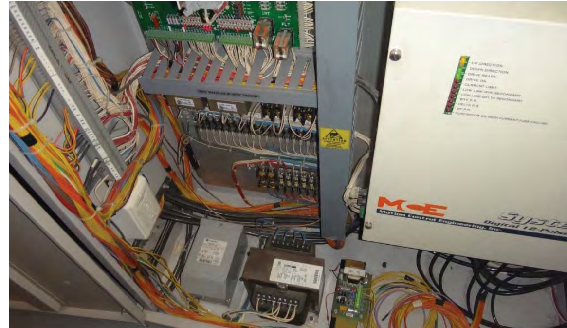
Figure 1 - Motion Control Engineering (MCE) IMC controllers with energy efficient 12 pulse SCR drives installed on Cars 1-10.
