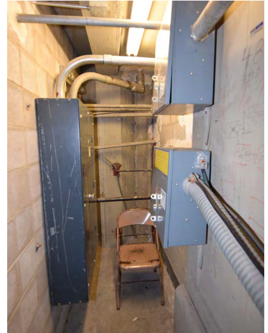
Electrical closet on upper level
