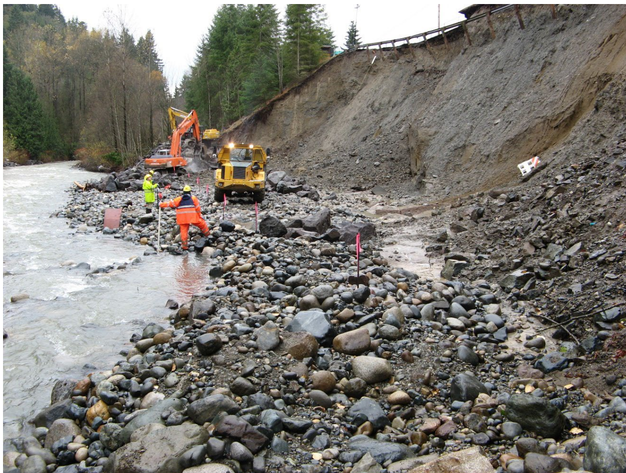
Upper Preston Road damage on the Raging River, November 2006
