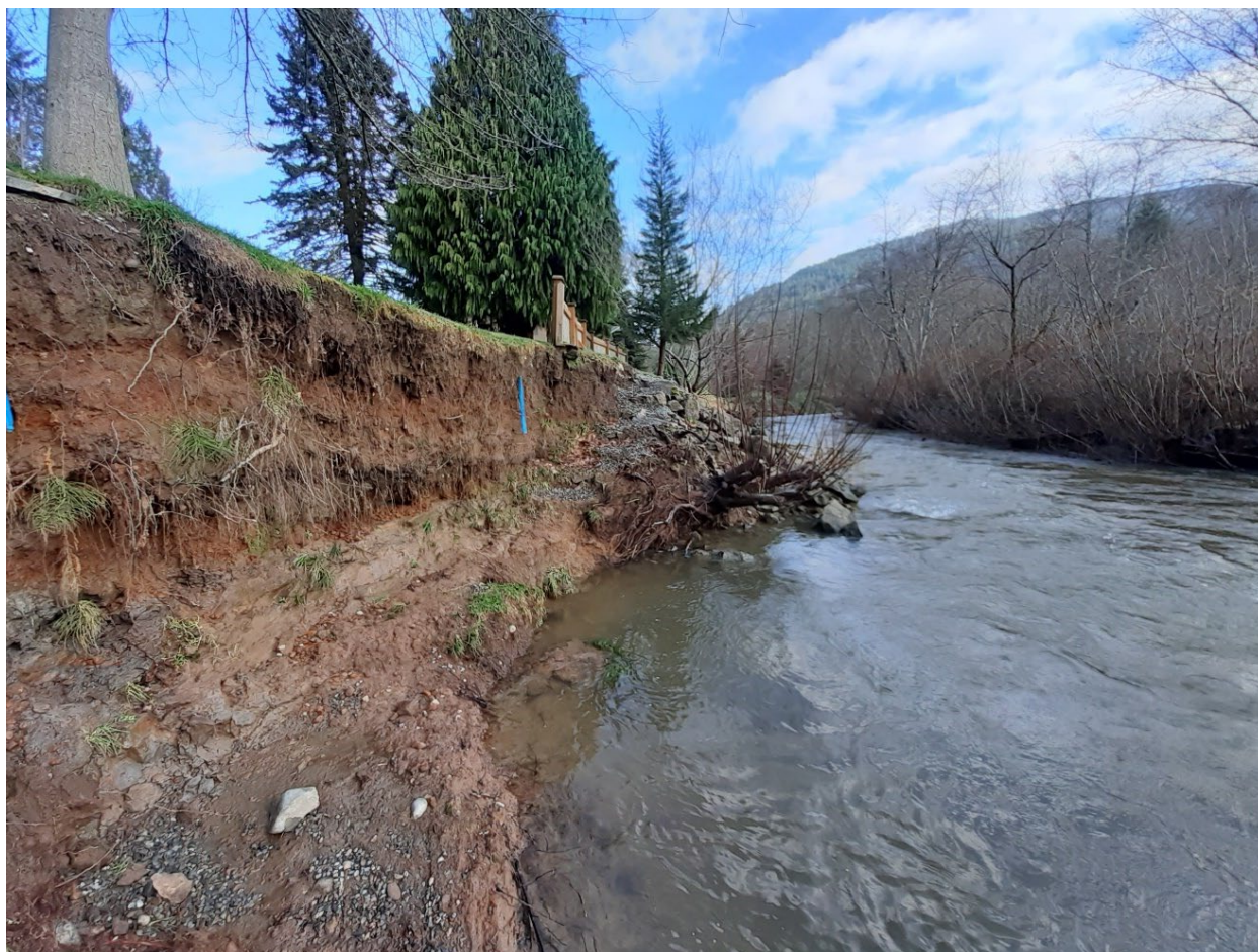
Erosion from Issaquah Creek flooding, January 2021
