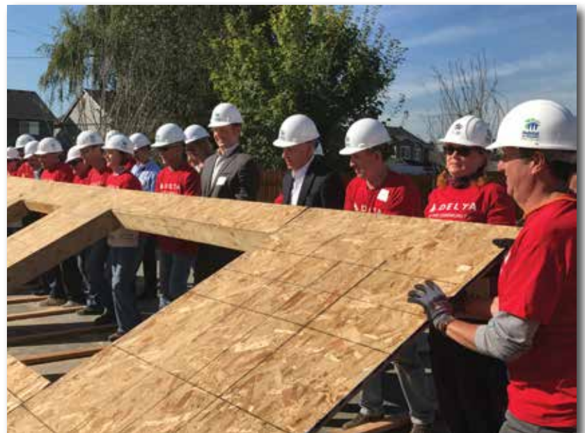
Raising the wall for one of nine Habitat for Humanity Blitz Build homes for veterans in Pacific.
