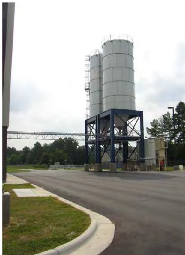
Typical: Product Storage Silos
