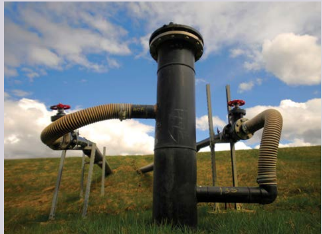
Part of the landfill gas collection system at the Cedar Hills Regional Landfill.
