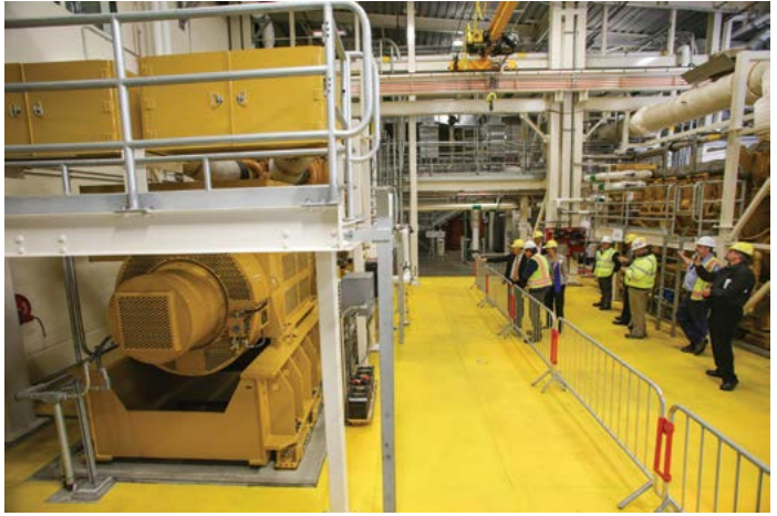
The cogeneration facility at the West Point Wastewater Treatment Plant turns digester gas generated during the treatment process into electricity, which is sold as green energy in partnership with Seattle City Light, and heat energy, which is used onsite.
