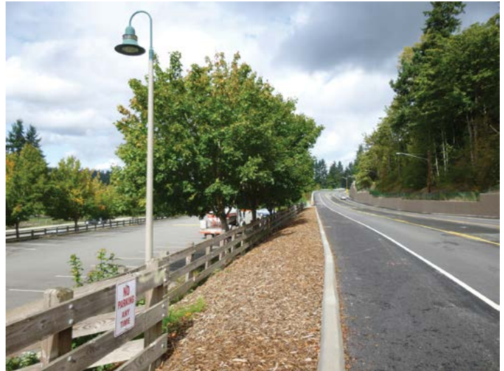
A stretch of NE Novelty Hill Road project near Perrigo Park that includes porous asphalt shoulders and Low Impact Development strategies.
