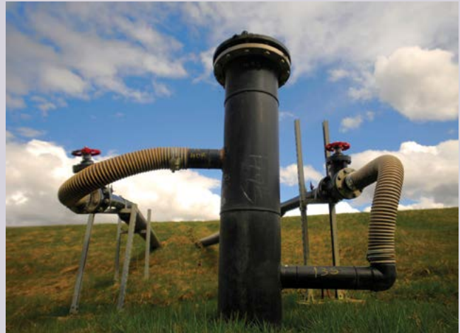
Part of the landfill gas collection system at the Cedar Hills Regional Landfill.
