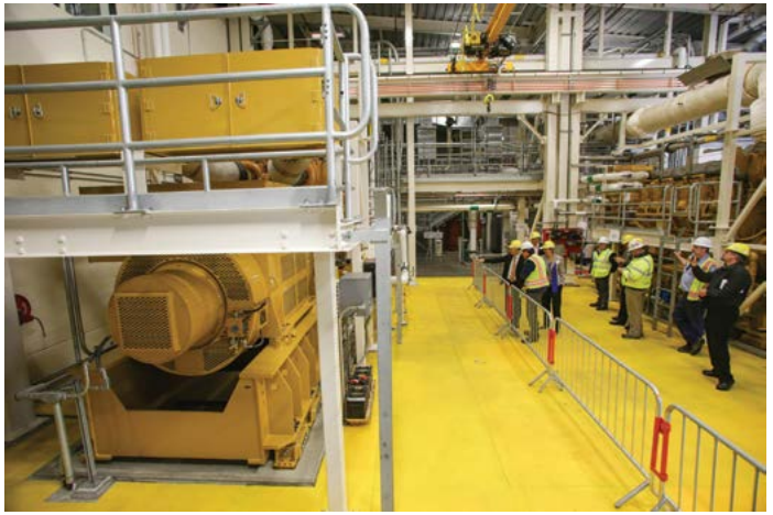
The cogeneration facility at the West Point Wastewater Treatment Plant turns digester gas generated during the treatment process into electricity, which is sold as green energy in partnership with Seattle City Light, and heat energy, which is used onsite.
