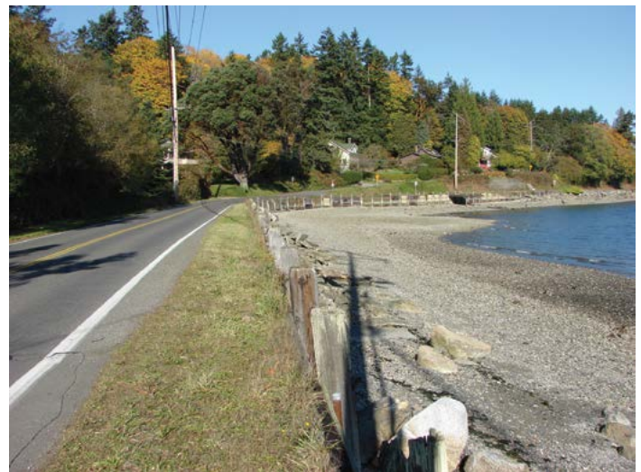
Dockton Road SW, located on Vashon Island in unincorporated King County, is protected by a 100-year old seawall that is vulnerable to storm surges and sea level rise.
