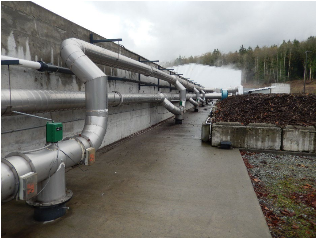
Figure 5-6. ASP air manifold, Lenz facility
