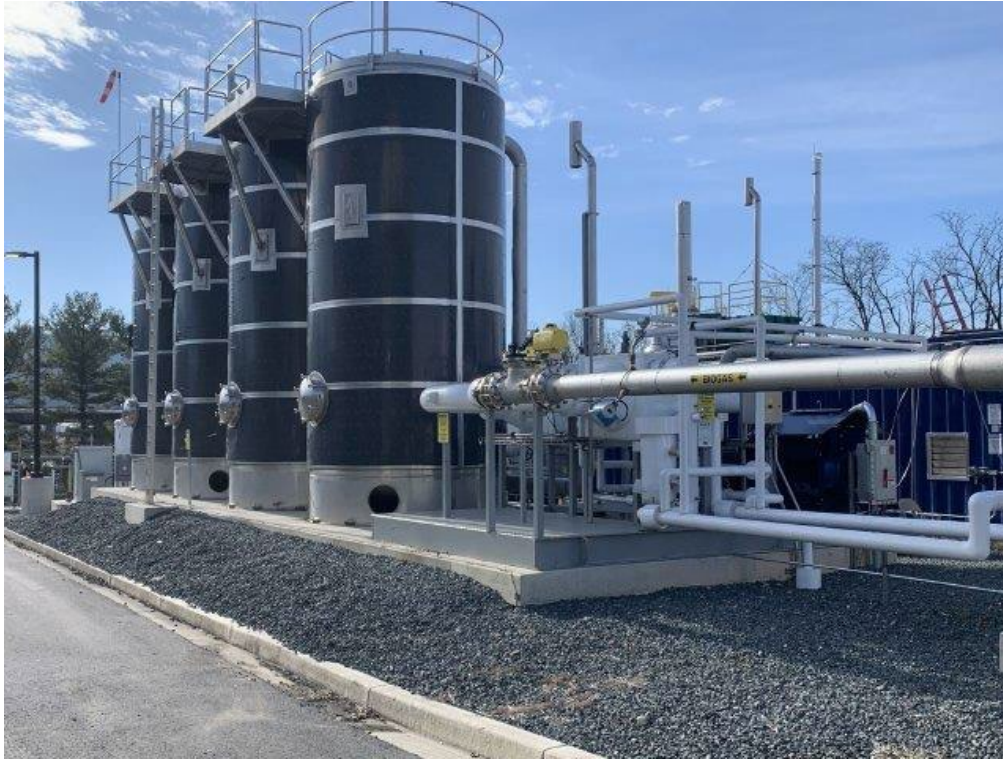
Figure 3-7. Biogas cleanup system at Bioenergy Devco AD facility
