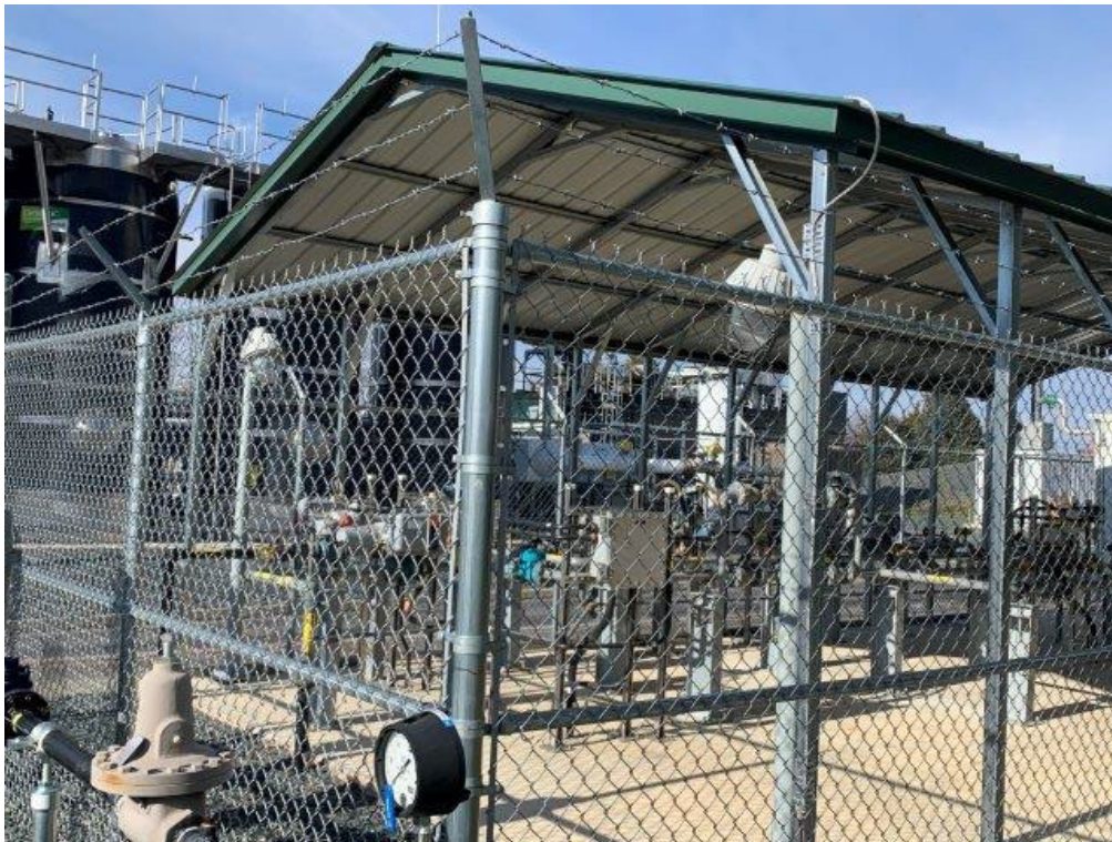
Figure 3-8. Gas testing and GC system at Bioenergy Devco AD facility
