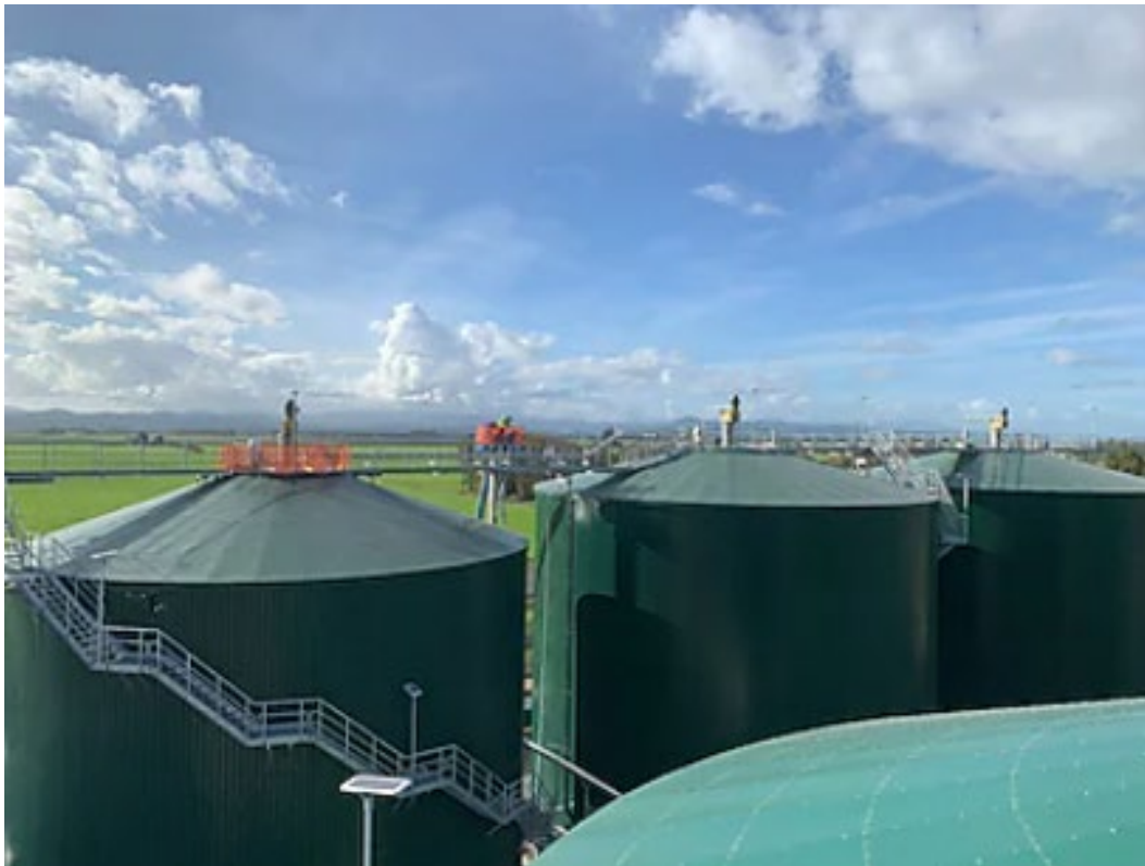
Figure 5-2. JC Biomethane’s anaerobic digestion facility in Junction City, Oregon
