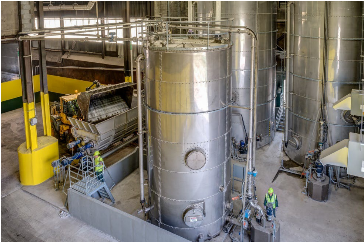
Figure 2-10. 250 tpd CORE system in New York City
