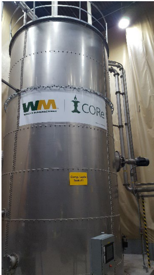
Figure 2-11. Receiving and feed-in station tank located adjacent to the NYCDEP WWTP anaerobic digesters
