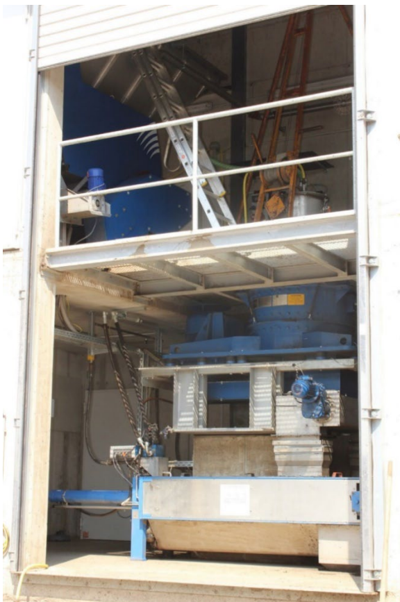
Figure 2-2. Fitec, Rothmuhle biogas plant in Germany: BioSqueeze unit
