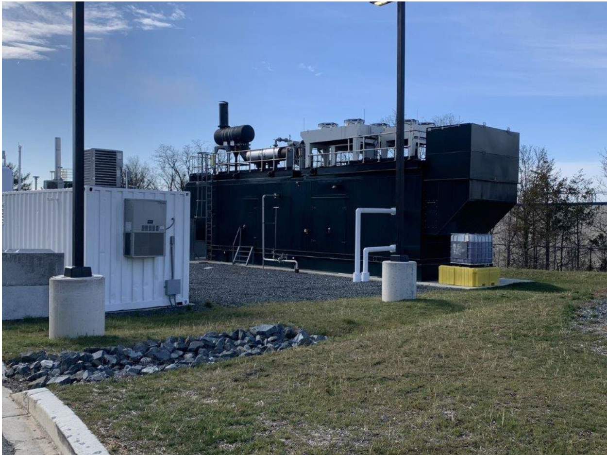
Figure 3-9. Combined heat and power unit at Bioenergy Devco AD facility
