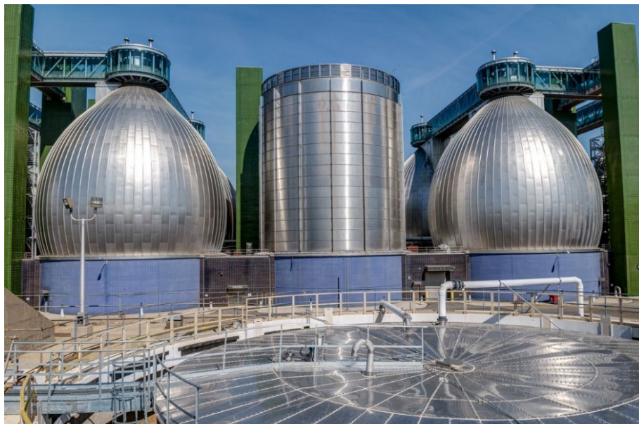
Figure 2-12. NYCDEP WWTP anaerobic digesters
