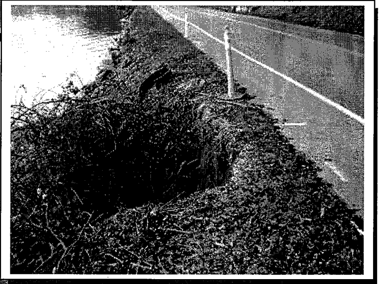
Typical void due to rock wall erosion.
