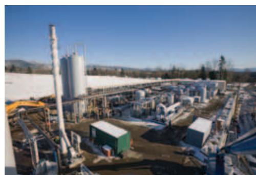
BioEnergy Washington’s renewable energy facility, fueled by landfill methane, at the Cedar Hills Regional Landfill
