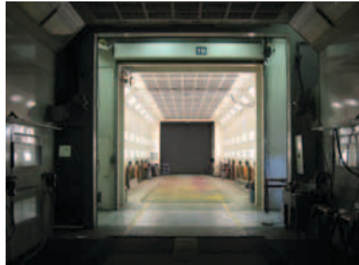
Lighting efficiency retrofit in a painting booth at a Metro Transit bus base
