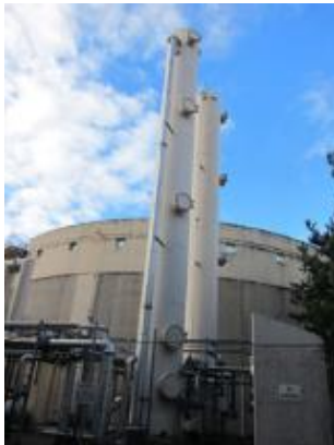
South Treatment Plant Produces biomethane
