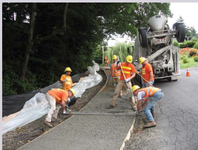
King County uses concrete for many types of projects and is exploring using low GHG emissions alternatives.
