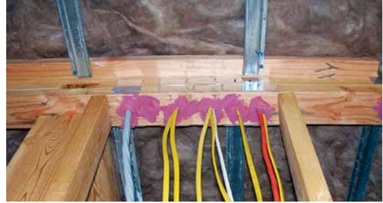
In an addition, new construction or a gut remodel, there are many opportunities to seal electrical penetrations and top and bottom plates. Source: O'Brien & Company
