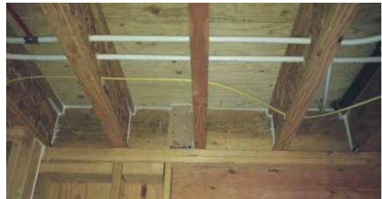
Air sealing with expanding foam or caulk at a rim joist is an effective means of sealing leaks. Source: O'Brien & Company
