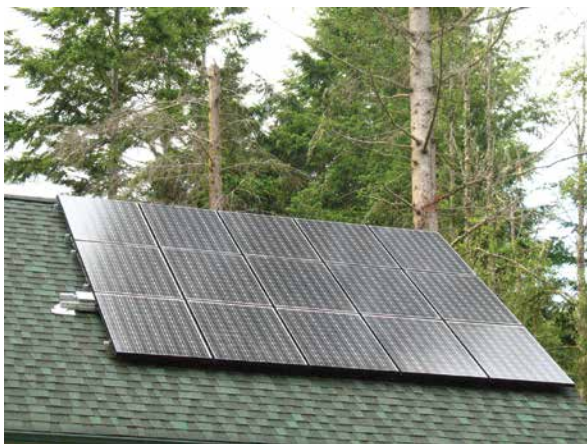
Composite Roofing with solar photovoltaic panels. Source: O'Brien & Company.
