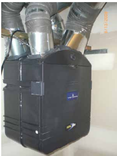
This is one example of a heat recovery ventilator located within a conditioned space. Source: O'Brien & Company.
