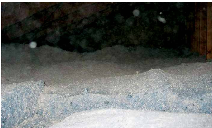
Any attic insulation should be smooth across the entire home. Mounding, lumps, valleys, voids and other problems with uniformity significantly reduce the overall R-value of the insulation. Source: O'Brien & Company.
