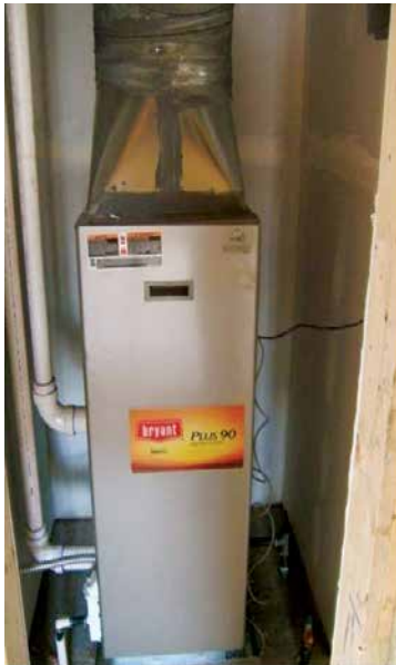
High Efficiency Energy Star Furnace with direct vent and condensate line. This furnace also includes ducted fresh air (not shown in the photo). Source: O'Brien & Company.
