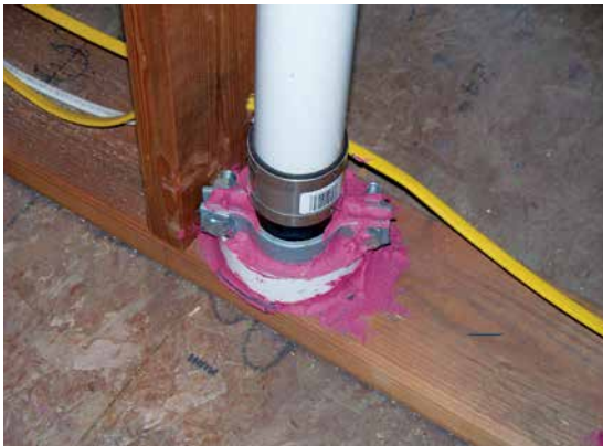
In a kitchen or bathroom remodel, or new construction, sealing plumbing penetrations is easy and effective. Source: O'Brien & Company
