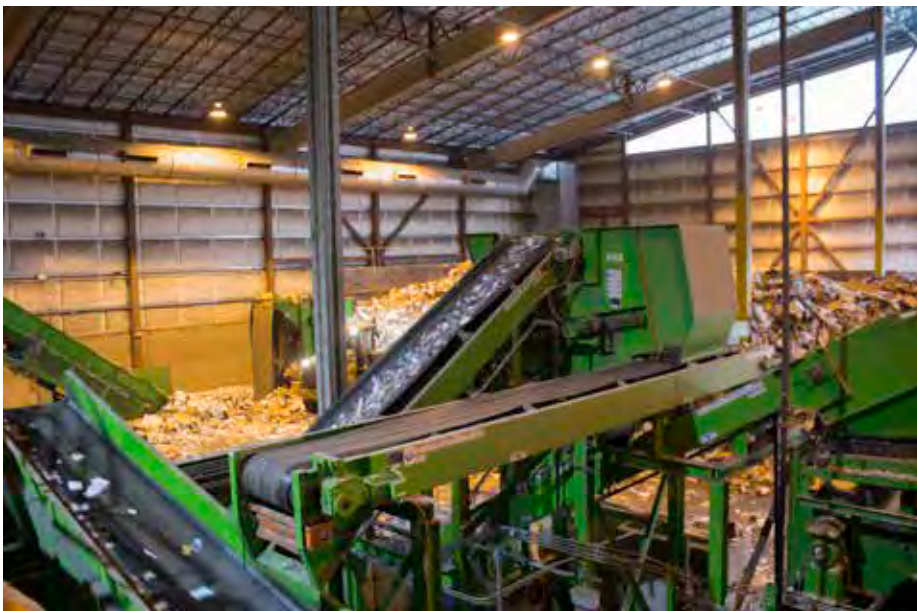
Recology CleanScapes materials recovery facility
